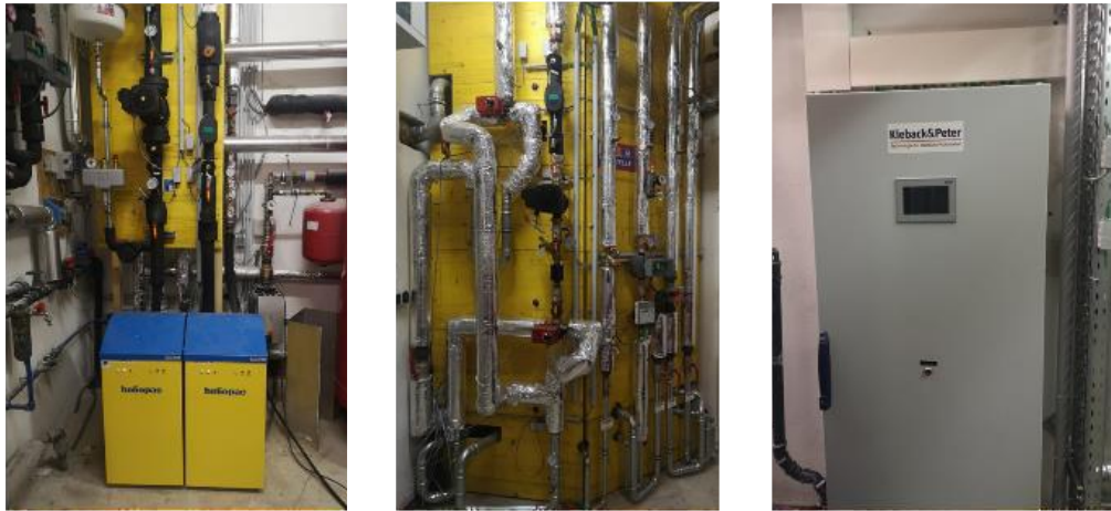
Figure 10: Pictures of the thermal equipment
