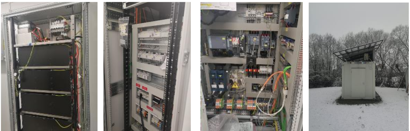
Figure 9: Pictures of the electric system container
